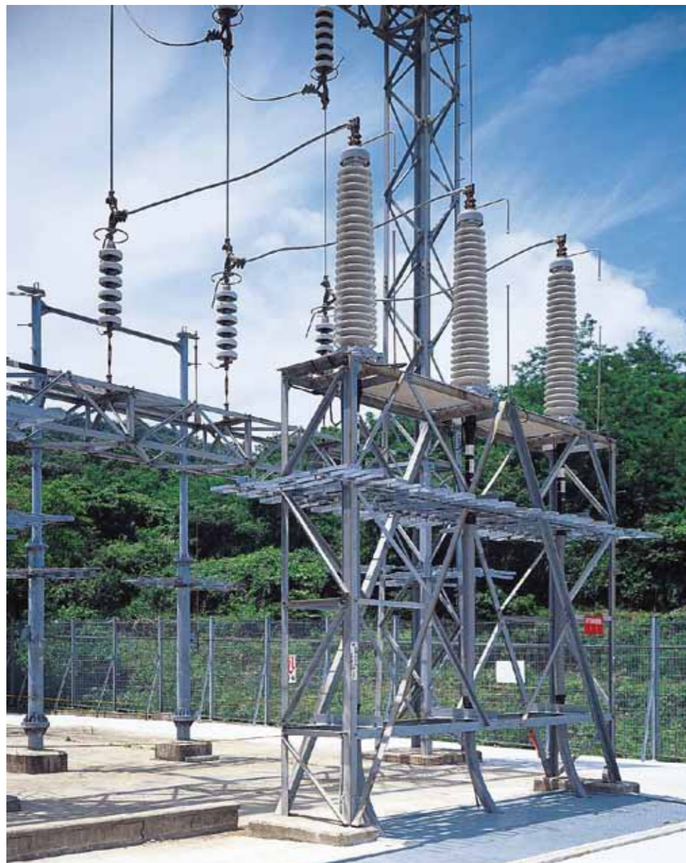
Installed outdoor sealing end
