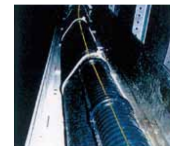
Cable temperature monitoring by Fiber-Optic Sensor
